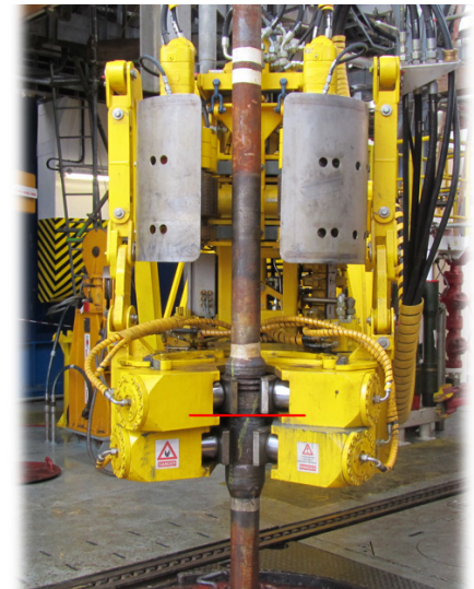
The image from the tool joint assist system indicates the current height configuration with a red line.
